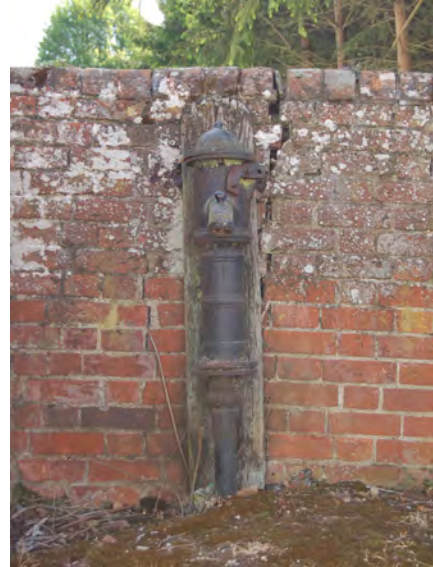
Picture 1.19 Any opportunity to repair the village pump would be beneficial.
